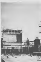
THE ANTILLES Chemical Company of February. Then an eight- to ten-heaters and flush all equipment to be anticipated to be the TERMINACION DI trabanon mesperá pa fin di Februari. Despues lo catalyist, pa seca e heaternan y lab limpi. E fecha pa cuminsa operacion
